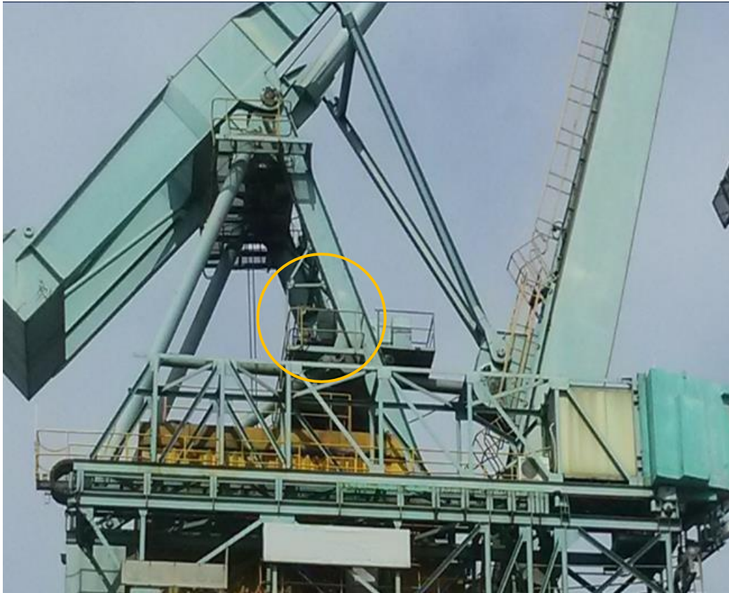
Operating motor at LLC Luffing
