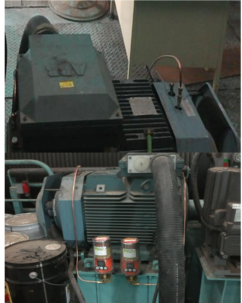
Remote installation with copper tubing due to vibration
